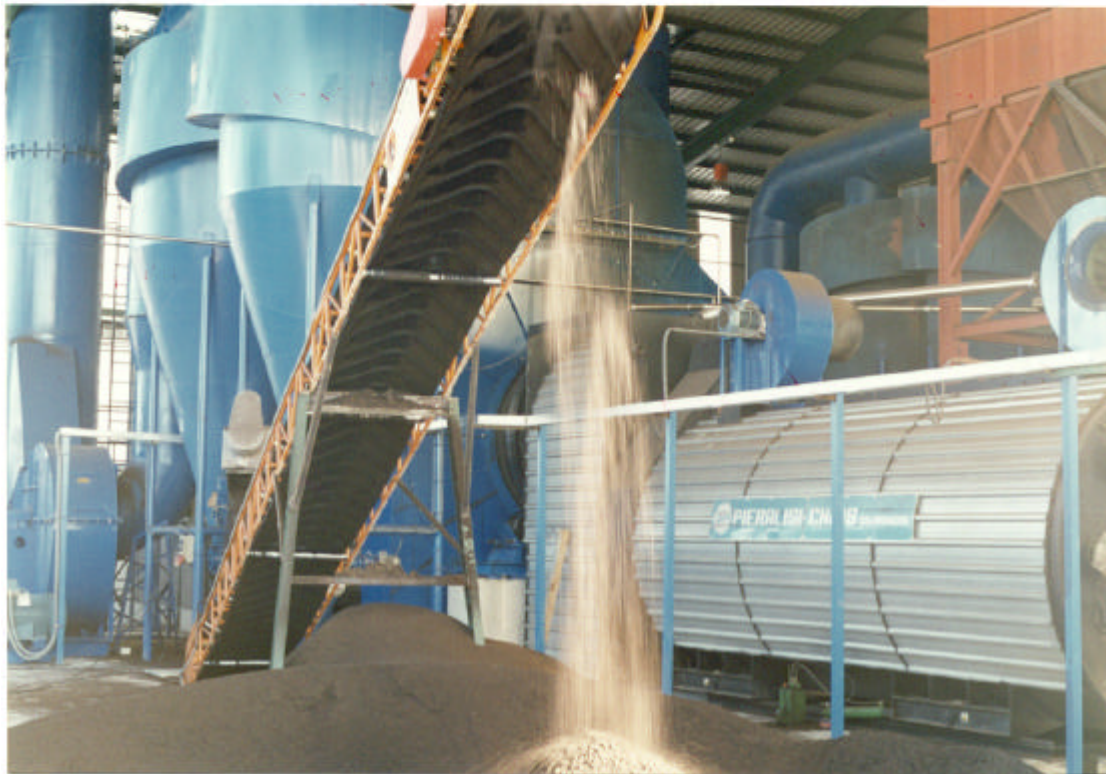
La Gineta plant (Albacete) – Dryers
