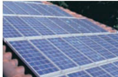
→ Discreetly blending in with roof tiles, solar panels offer numerous advantages. www.ata.org.au/basics/bassolar.htm
