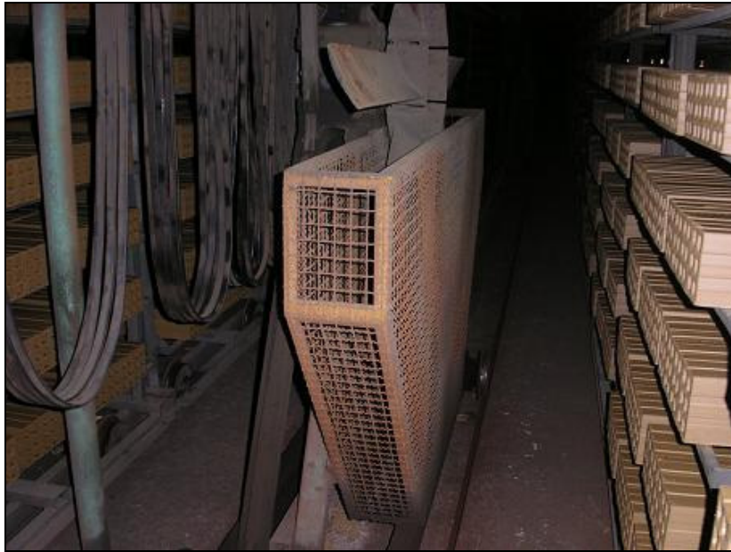
Image 3.8: Fans for the movement of air within the dryer
