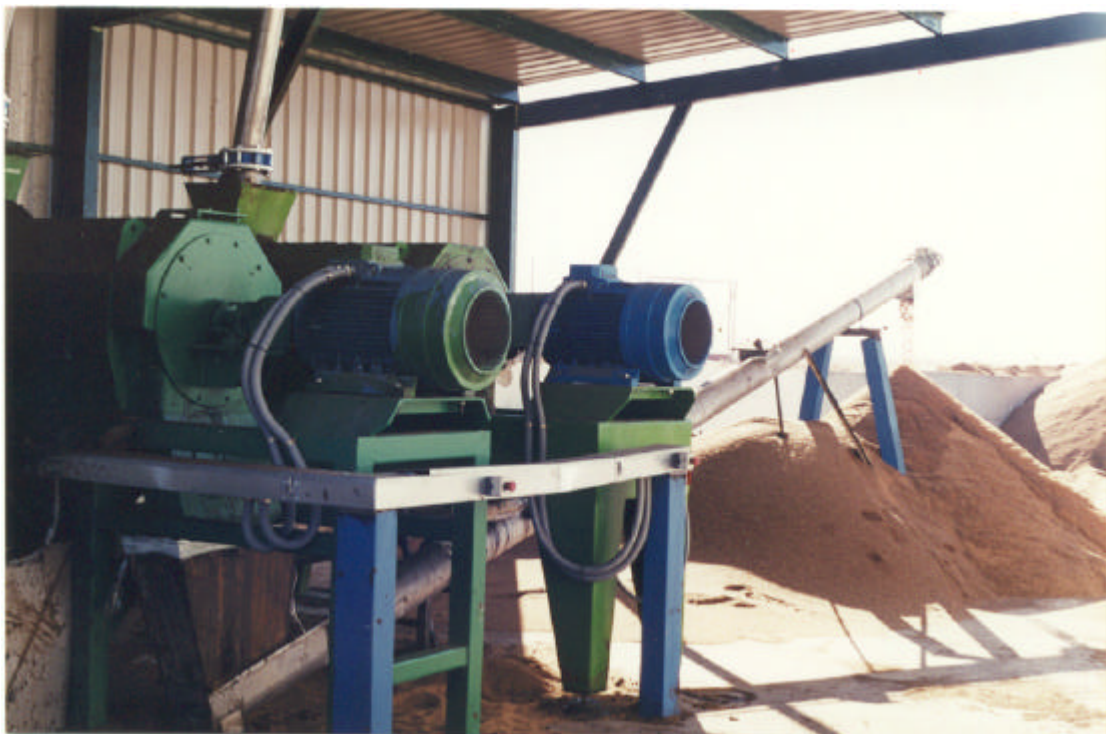
“La Gineta” plant (Albacete – España) Separation equipment of the stones from the spent olives
