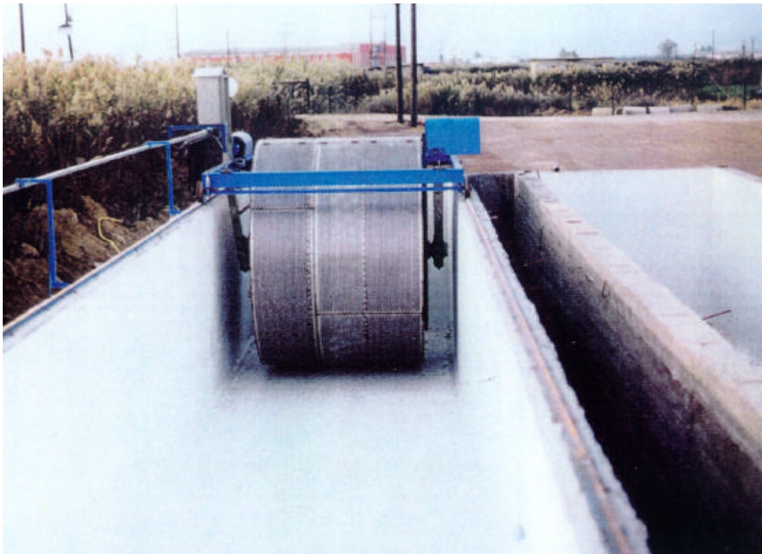
Kalamata plant, Greece (Life project 1995). Rotational speed : 6 rpm. Lineal speed: 1.8 m/min. Tank length : 25 m. Capacity : 100 m 3
