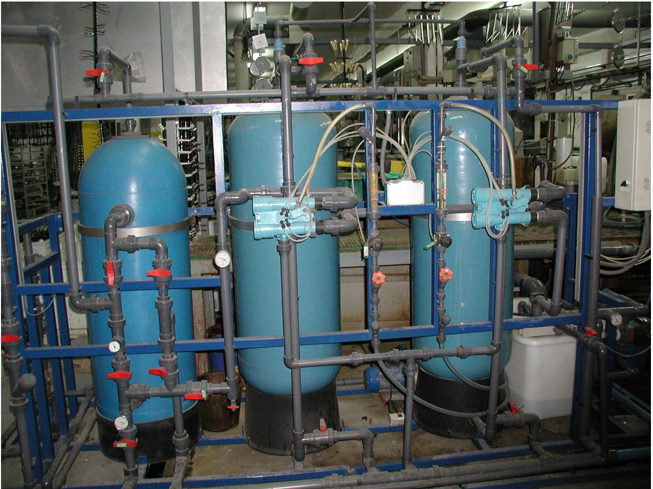
1 – Recycling equipment for water used for washing with ion-exchange resins.
