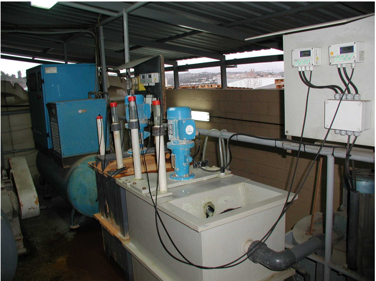
8 – Installation for the oxidation of cyanides, before the evaporation of the wastewater.
